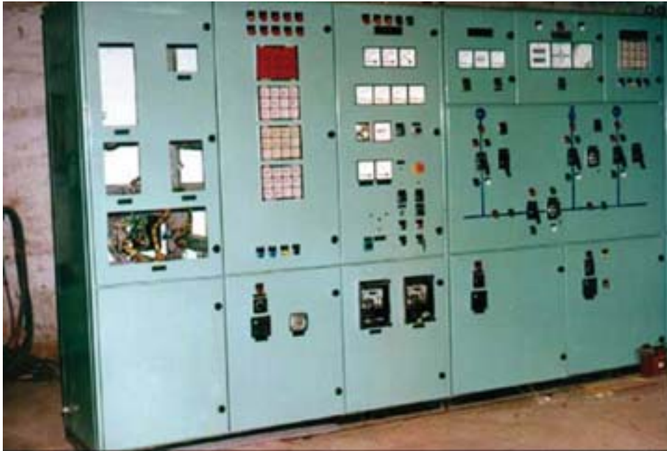
Power Factor Improvement
