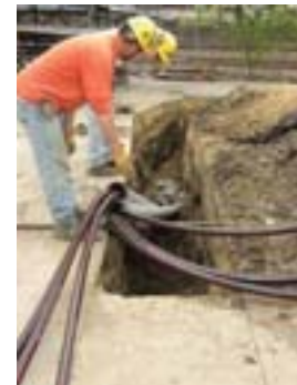
Underground transmission system.
